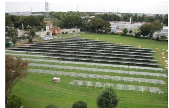
Installed solar panels on plant premises
